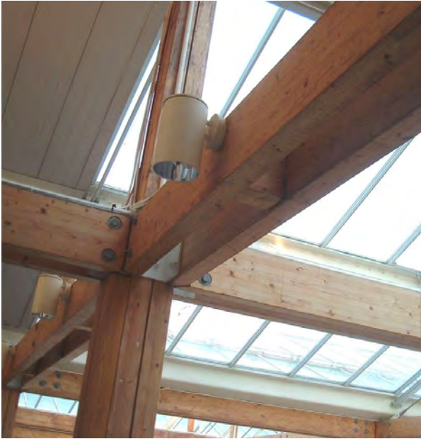
Figure 6. Gluelam structure in the Portland Building, University of Portsmouth, United Kingdom (Wikipedia).
